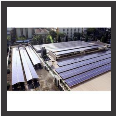
Solar Grid Tied Systems For Industrial
